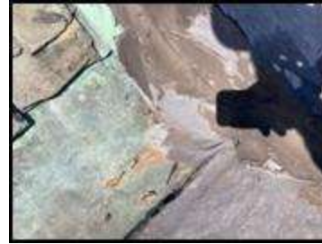
Crack at roof juncture 10-26-22.
